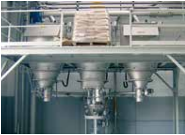
Additives metering & weighing
